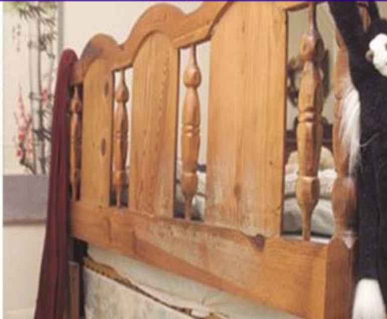
Mold growing on a wooden headboard in a room with high humidity.
