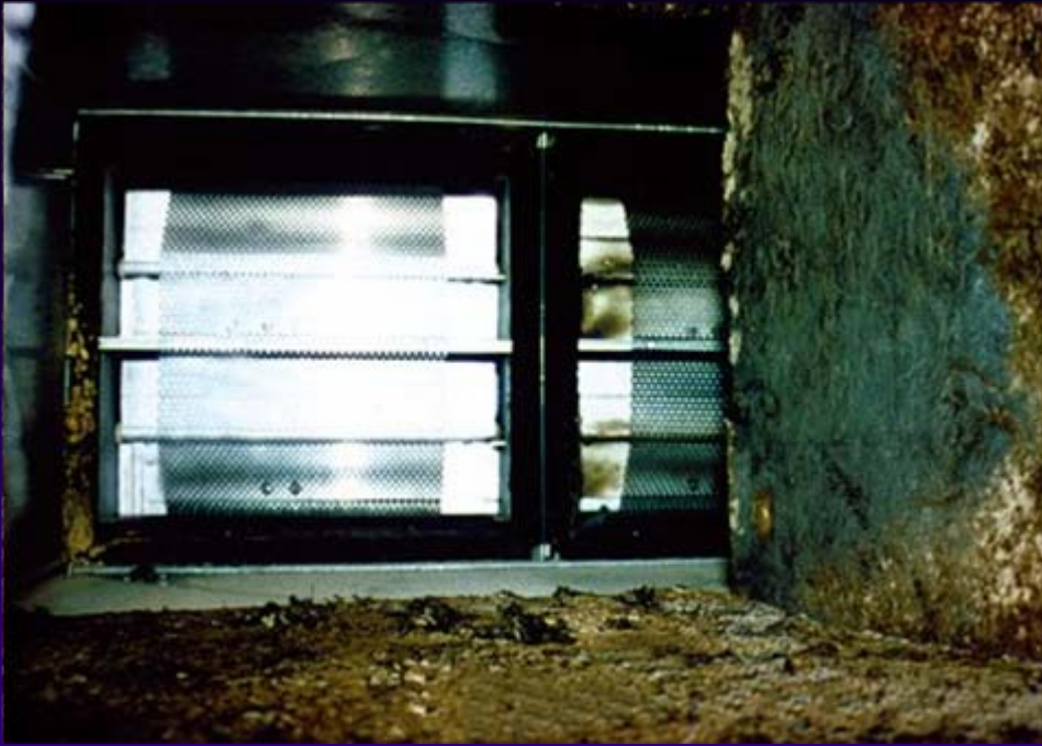
Moldy Duct Work
