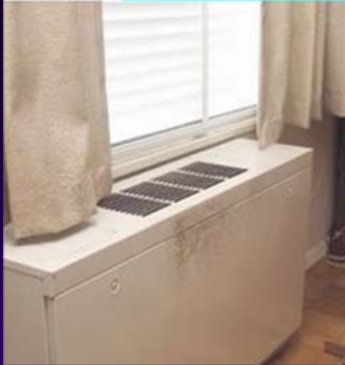
Mold growing on the surface of a unit ventilator.
