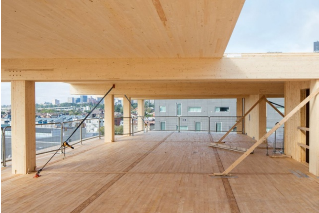
Construction using CLT at the Arbora Complex in Montreal, Quebec. Source: Nordic Structures
